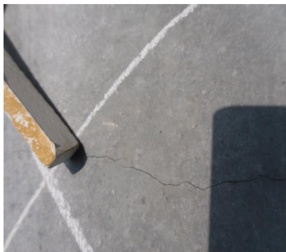
Fig. 4: Photograph showing Crack after application of Load Greater than Design Load.
