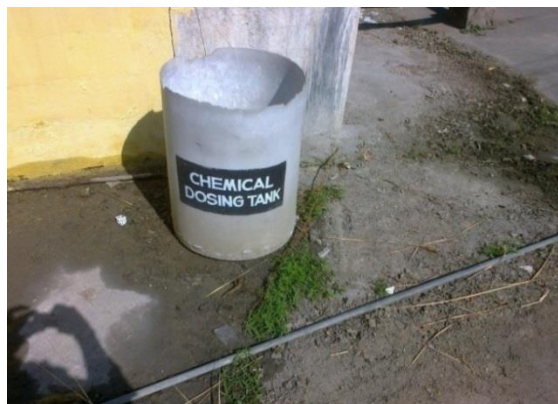
Fig. 7: Chemical Dosing Tank.
